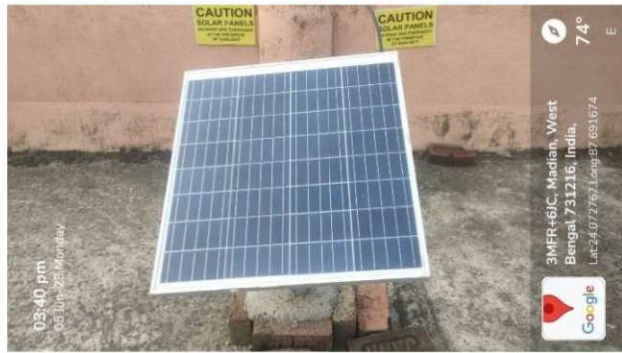
Figure 1e: The solar panel of figure 1c. The panel is fixed in the roof top to perceive sufficient sun light.
