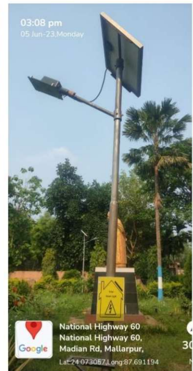
Figure 1e: The street light has been installed inside the Butterfly Garden situated in front of the institution.
