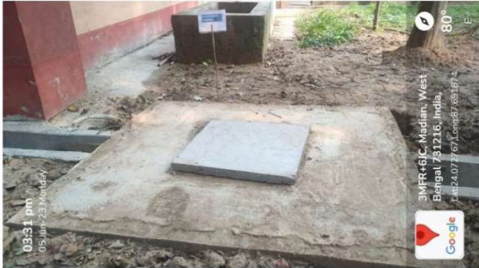
Fig 1: Ground water recharge chamber constructed in Medicinal garden area which is in west side of campus.
