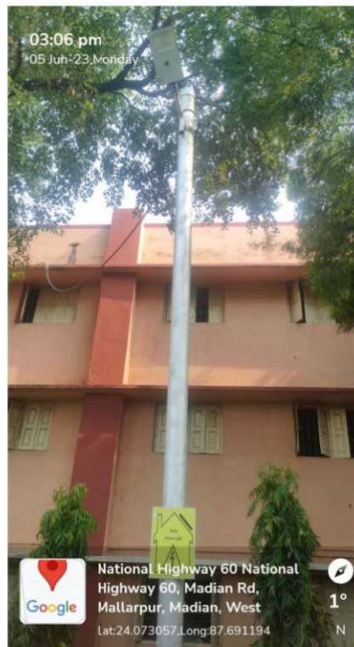
Figure 1d: The street light has been installed in the South-West side of the institution in front of the canteen building.
