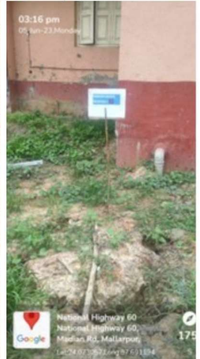
Fig 6: One of four soak pits for roof top water and sewage of boys' toilet constructed in east side of the campus.
